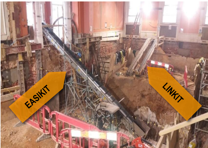
Pictured in this basement excavation are the EASIKIT modular conveyor (center) and two LINKIT portable conveyors (center, right). The EASIKIT system was used to excavate material, the LINKITs to place new material.
